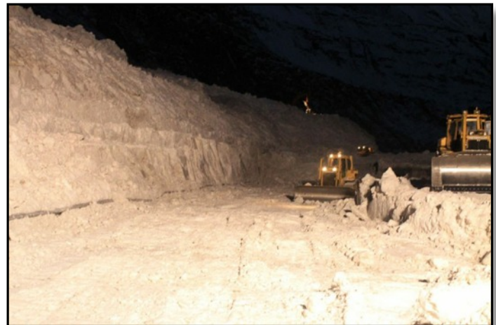
Beginning on January 24th, massive avalanches occurred throughout Thompson Pass/Keystone Canyon on the Richardson Hwy. The debris blocked a 50 some mile section of the roadway from Mile 12-64 with debris that measured 20-50' deep. DOT began the nearly 2 week process of clearing the highway before it was once again open to traffic to and from Valdez.
